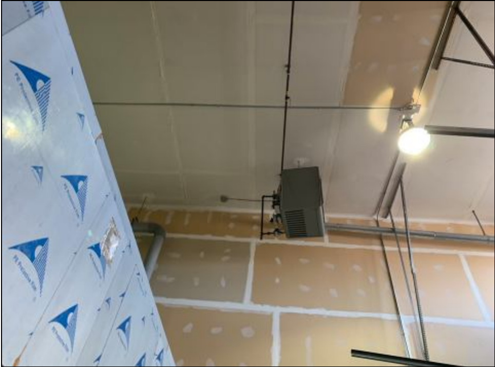
Overhead space heater
