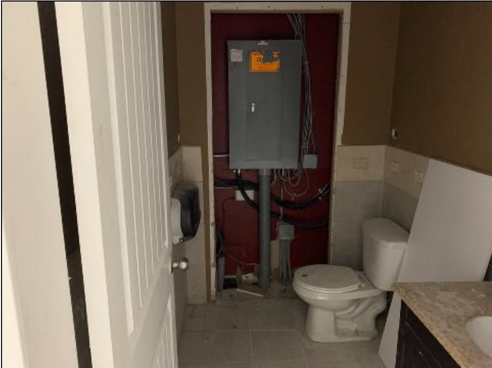
Electrical and washroom
