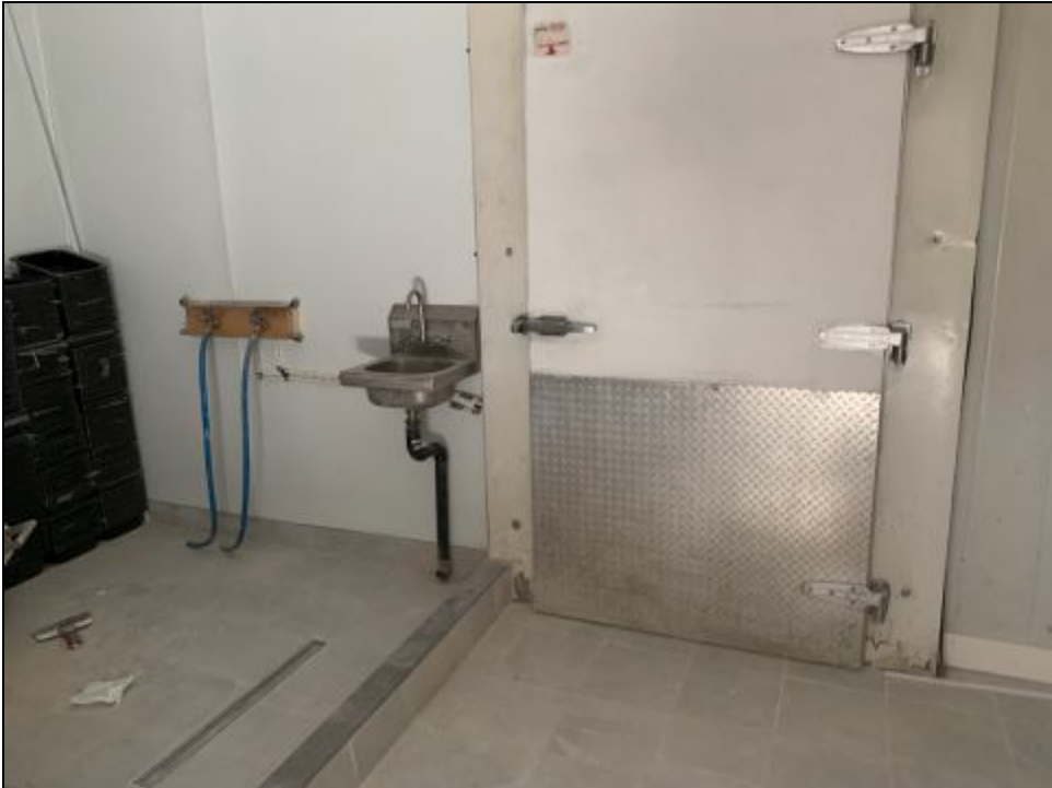
Walk-in cooler entrance
